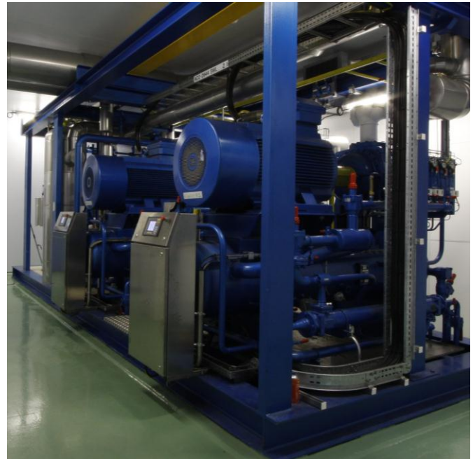
Two Vision280™ OPLCs Controlling 2 Large Ammonia Compressors
